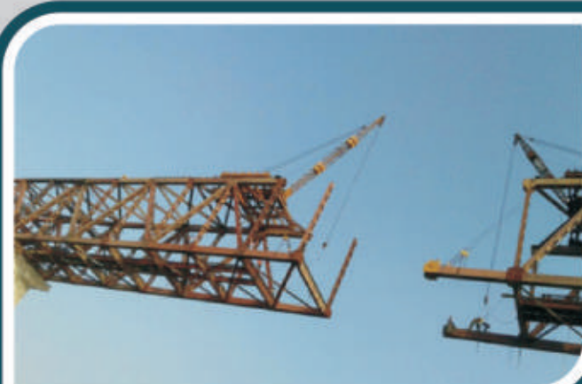
120 M Open Web Girder launching by Centre Closing Method at Baluaghat, Varanasi over River Ganga
