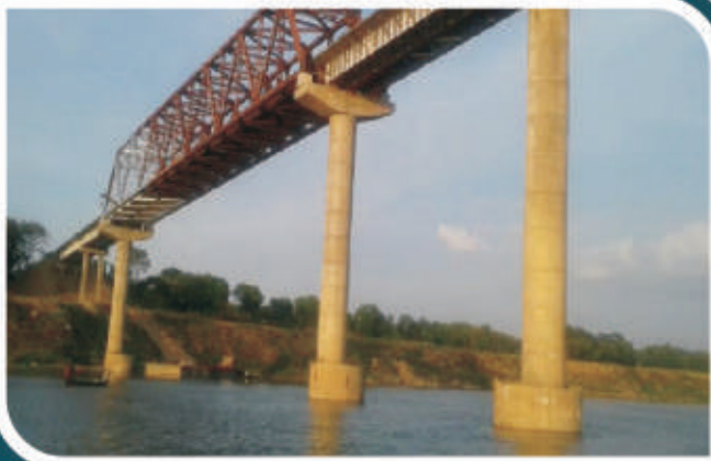
Fabrication and Erection of 90 mtr span Open Web Girder, 3x30 mtr Composite Girders over river Ganga over road bridge
