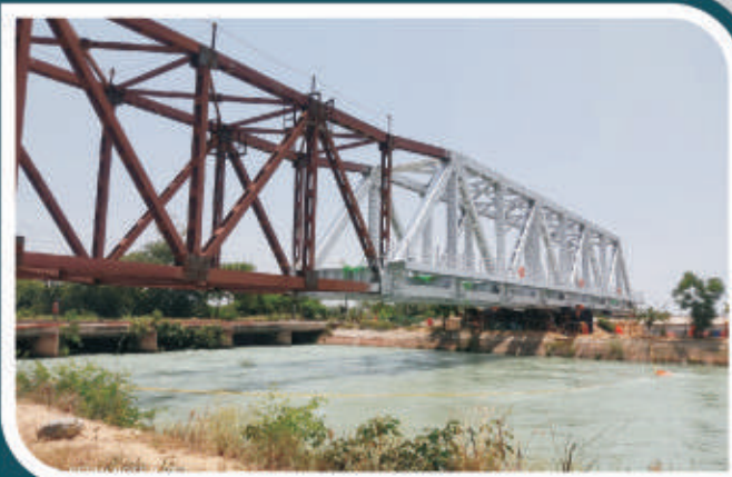
61 M Span launching over Sirhind Canal Punjab, by pulling Method (DFCCIL Project)
