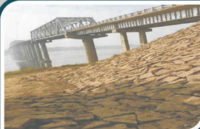
Completed ROB with Steel OWG of spans 72 mt x120 mt x72 mt
