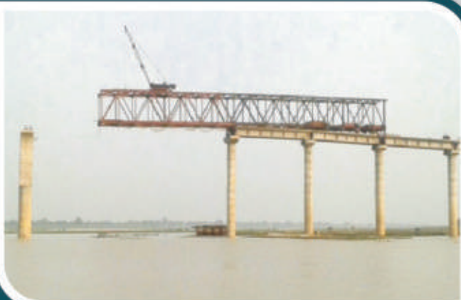
Erection by Cantilever Crane over Rivers, Spans of 120 mtr, 90 mtr, 72 mtr and 30.5 mtr ROB
