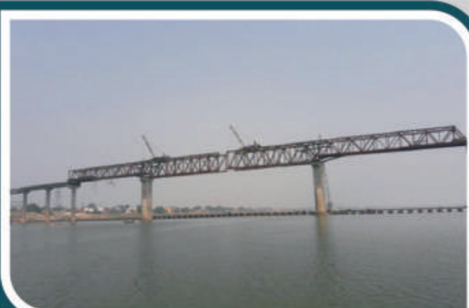
120 M Open Web Girder launching by Centre Closing Method at Samneghat, Varanasi over River Ganga
